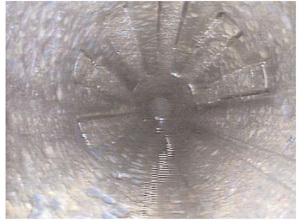
(Above) The camera reveals several slots cut in well casing during a RMOTC test project.
